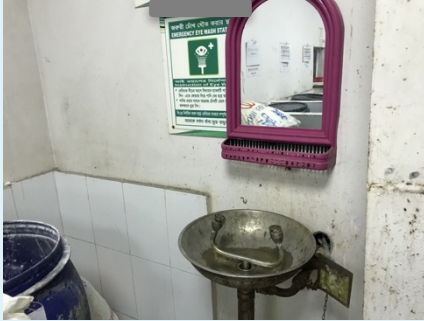
Improved Health & Safety: Installed eye wash station in the lab
